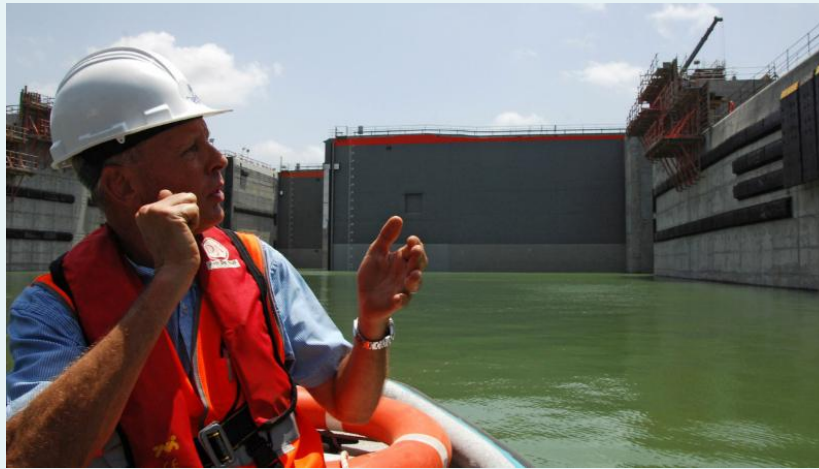
The Cocoli lockgates are tested during the Panama Canal expansion on July 3_ 2015. Photographer_ Ed Grimaldo_AFP via Getty Images
